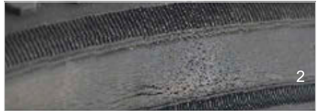
Figure 200: Examples of fatigue cracks (1) and ageing cracks (2)
